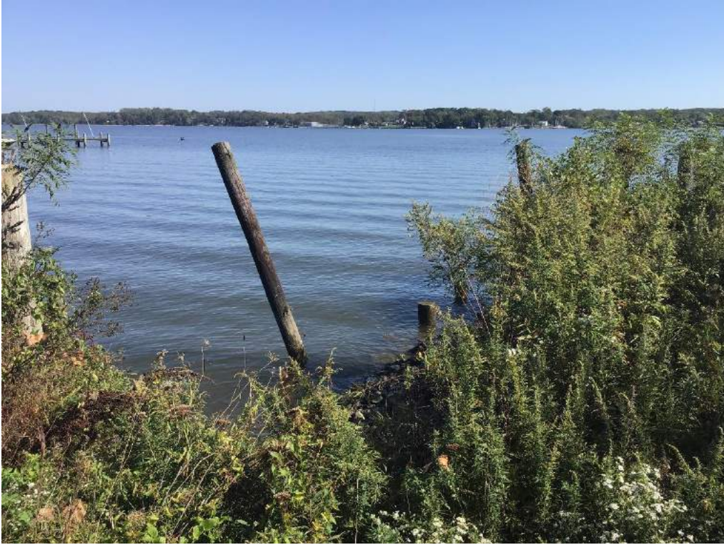
Photo 5: Eroded area where only the wooden piers remain
